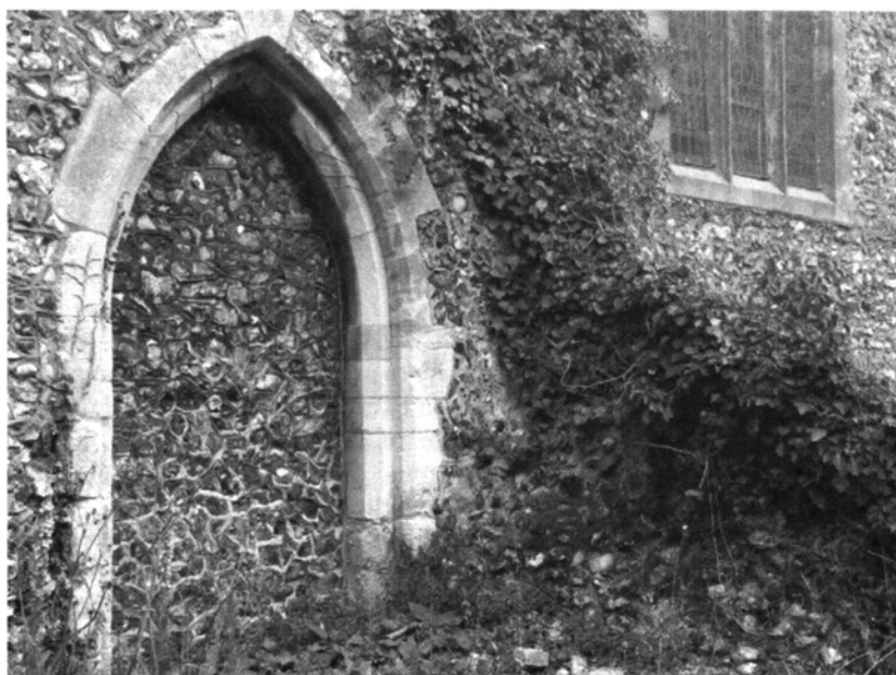
Ruined wall and blocked doorway leading to the south aisle of the church, marking the former passageway between the church and the west range of the college.
